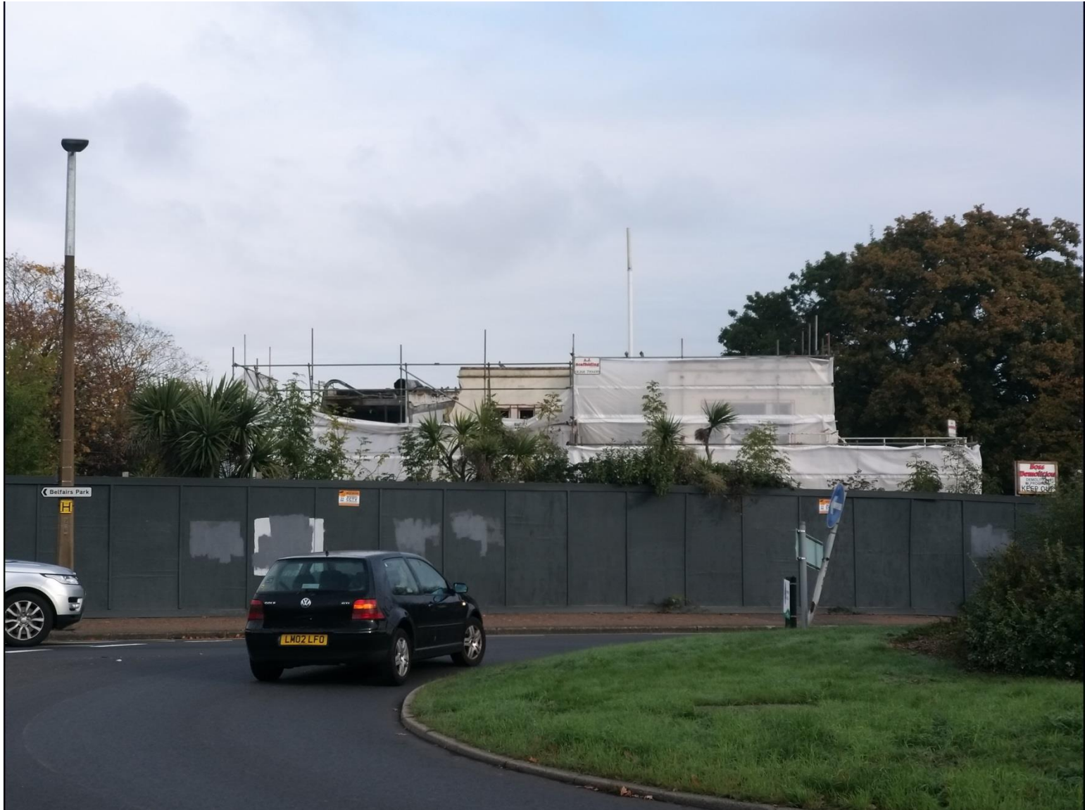
View of site from Eastwood Road
